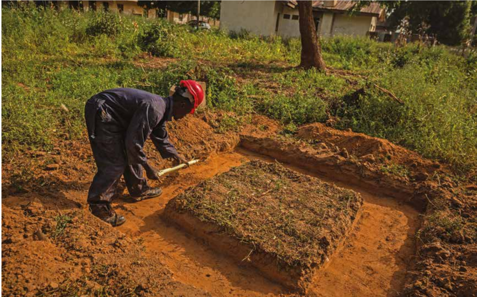
Workers at work in the area destined to become the distribution point for supplying drinking water to animals in Potiskum, Yobe State.
